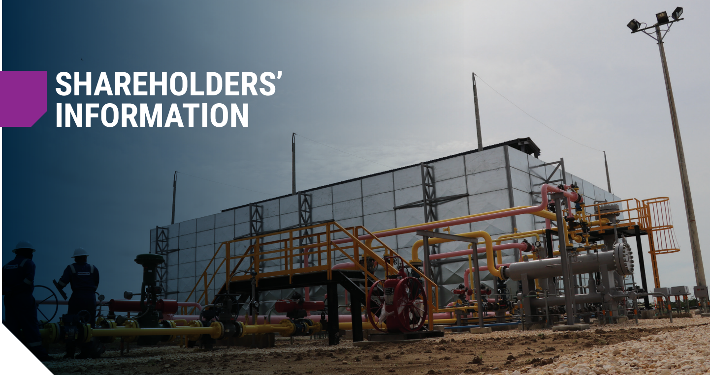
42 mmscf/d natural gas compressor station, Colombia.
